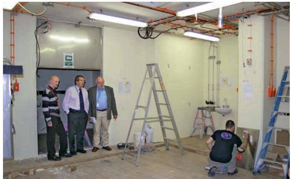
Left to right: Andrew Munro, Department of Innovation, Industry Science and Research (DIISR), AAHL Director Martyn Jeggo and Allan Kershaw, NCRIS Construction Project Manager, inspect the works.
